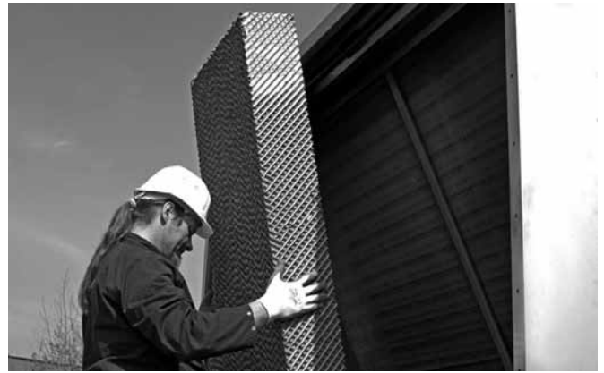
Figure 21: Removal pre-cooling media
