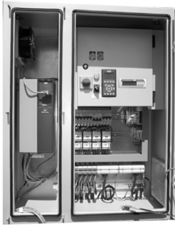
Figure 2: Control Panel with Variable Frequency Drive
