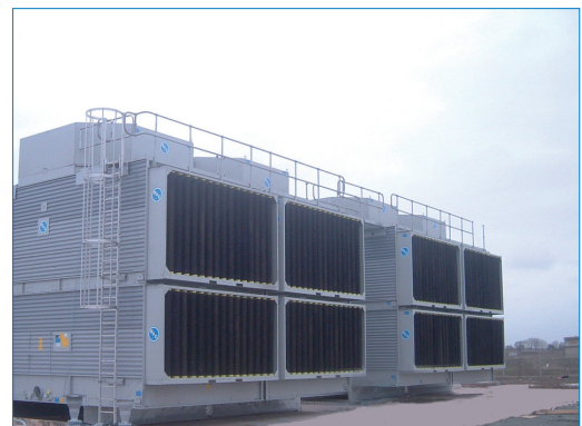
Figure 11: Intake and discharge sound attenuation on a BAC Axial Fan Open Cooling Tower
