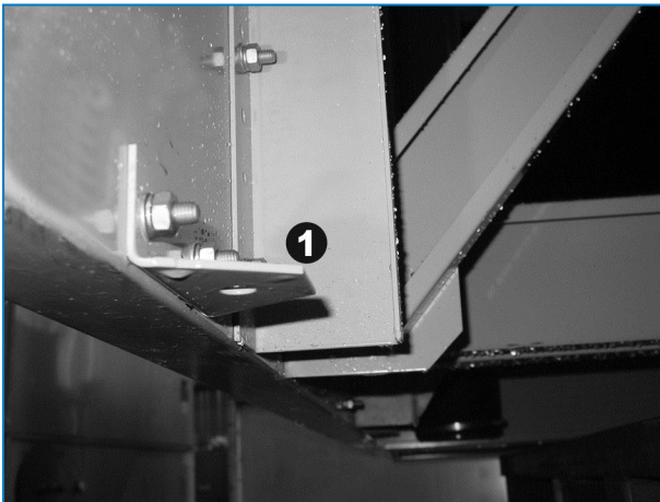
Inside View Plenum Section
