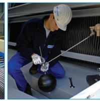
on site services
