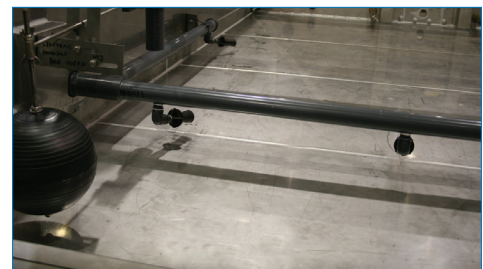
Cold Water Basin with Sweeper Piping
