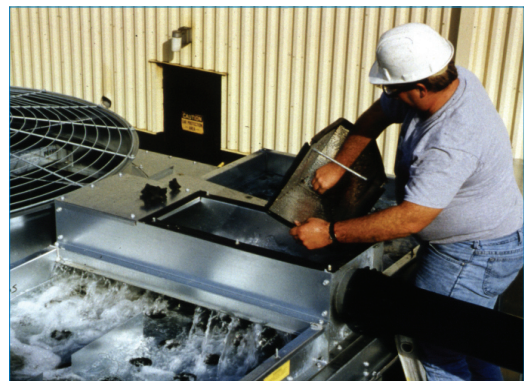
Hot Water Basin Strainer Cleaning
