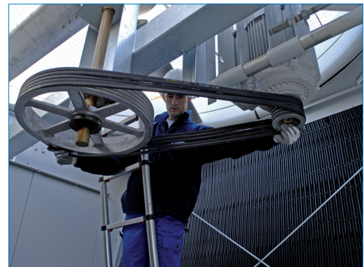
Mechanical Belt Drive System
